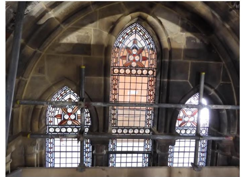
5.46 View of leaded lights re-fitted in level 2 corridor from Princess St courtyard
